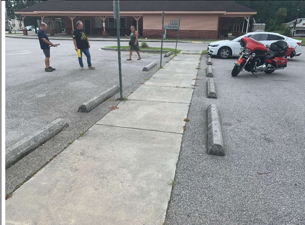
Parking area needs re-striping and the addition of a handicapped parking spot that is specifically van accessible.
