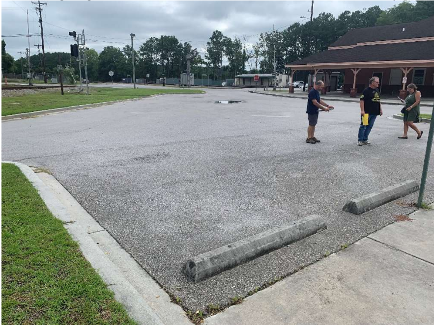
Parking lot requires re-stripping
