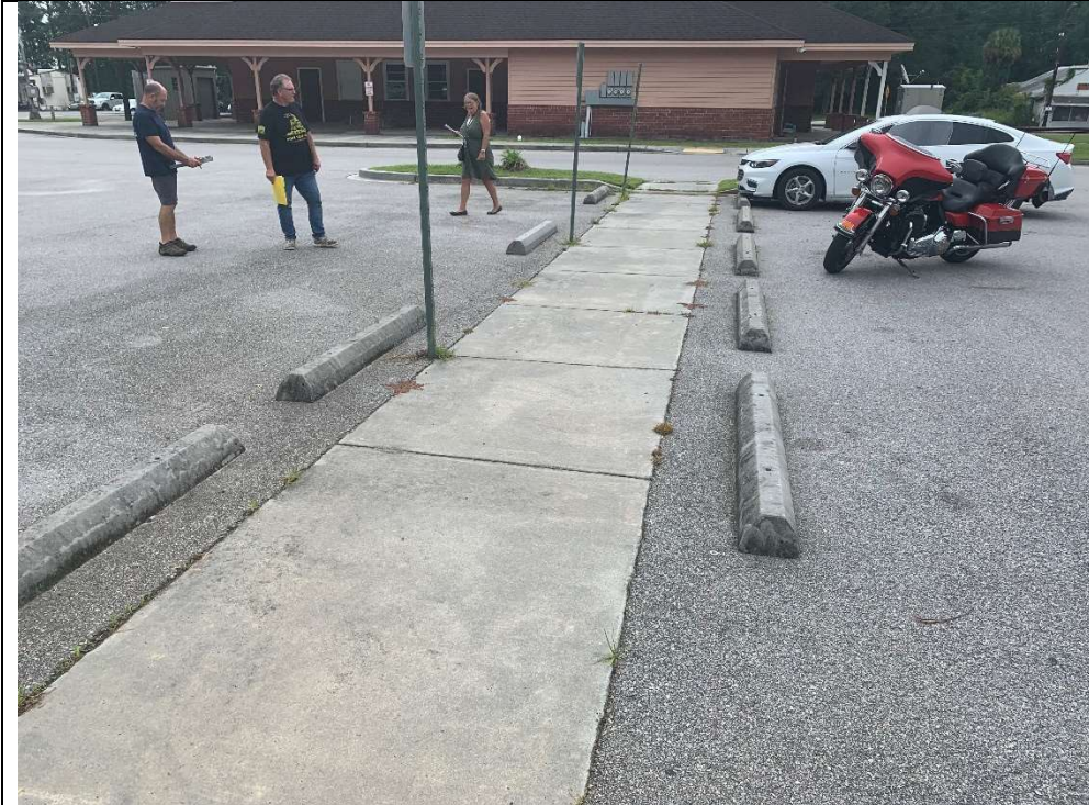
Parking area needs re-striping and the addition of a handicapped parking spot that is specifically van accessible.
