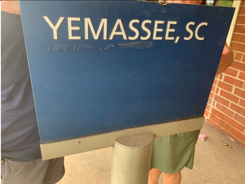
Braille signage has been filed down and needs to be replaced.
